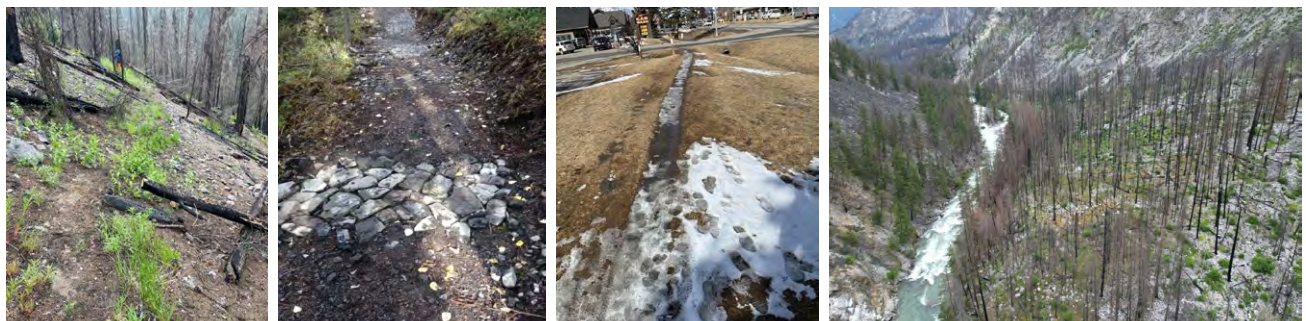
Figure 1. Sloughing, Rock Armouring, Freeze Thaw Environments, Burn Scar (from left to right)
