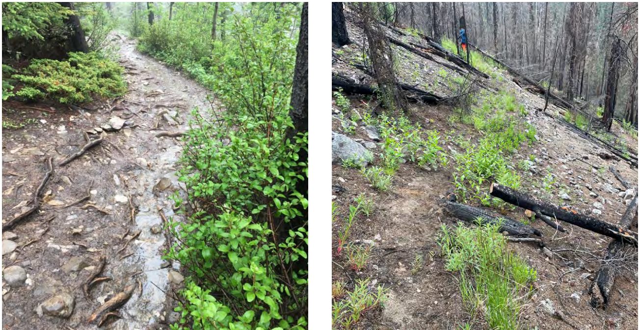
Figure 4. Cupped and Channeling (left) Sloughing (right).
